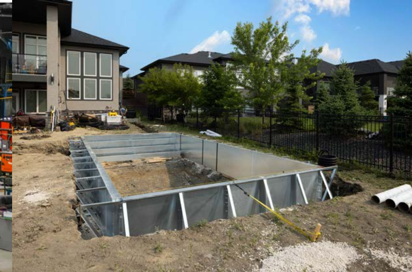
Ground-level view of a 14' x 28' steel pool kit in construction. The steel pool walls are 42" standard height panels, and there are alternating deck frames and X-frames with an open top 14' full-width step.
