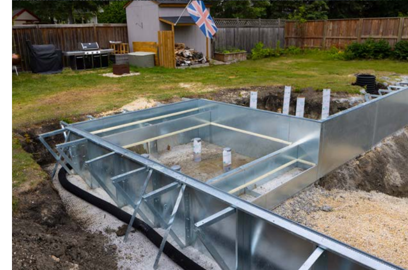
Ground level view of the 10' x 10' sun ledge/step combo on 42" G235 steel panels.
